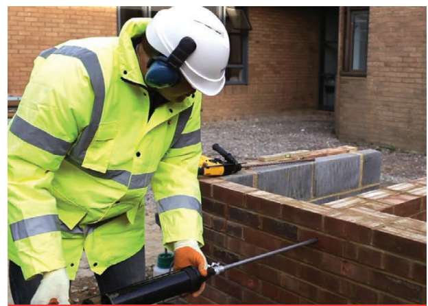
Inserting the grout-filled pinning nozzle, containing the CemTie, into the clearance hole
