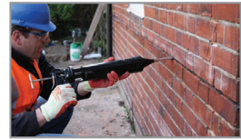
5. Insert a further bead of HeliBond over the exposed HeliBar, finishing 1/2" from the face, and 'iron' into the slot using the brick jointer.
