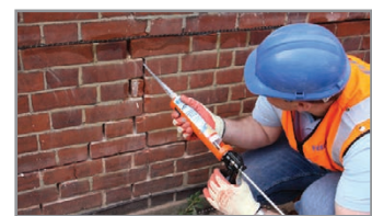
6. Re-point the mortar bed and make good the vertical crack with CrackBond TE3.
