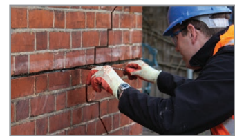
4. Using the brick jointer, or similar, push one HeliBar into the grout to obtain good coverage.
