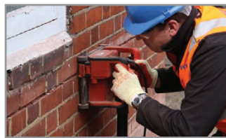
1. Rake out or cut slots into the horizontal mortar beds, a minimum of 20" either side of the crack.
