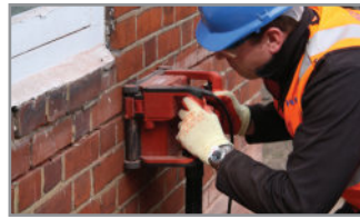
1. Rake out or cut slots into the horizontal mortar beds, a minimum of 500mm either side of the crack
