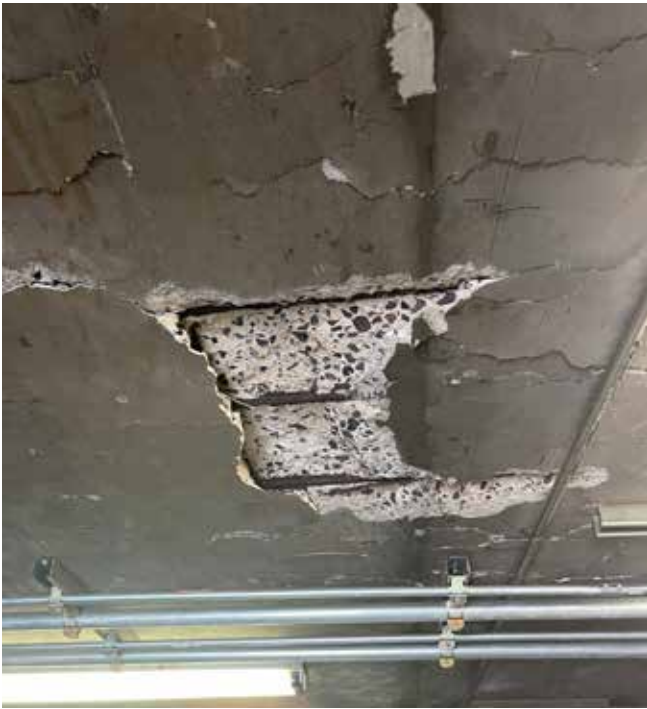
Elevator machine room ceiling damage
