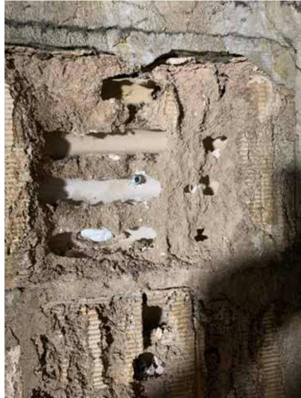
Damage caused by improper anchor installation
