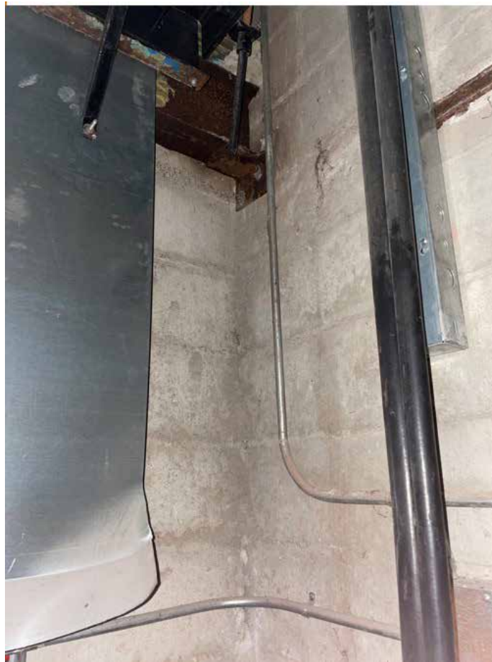
Water-damaged shaftway after repair
