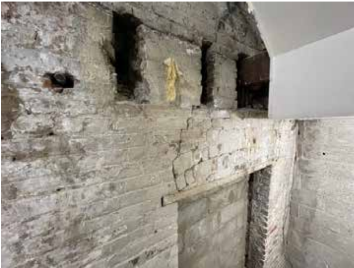
Water-damaged shaftway before repair
